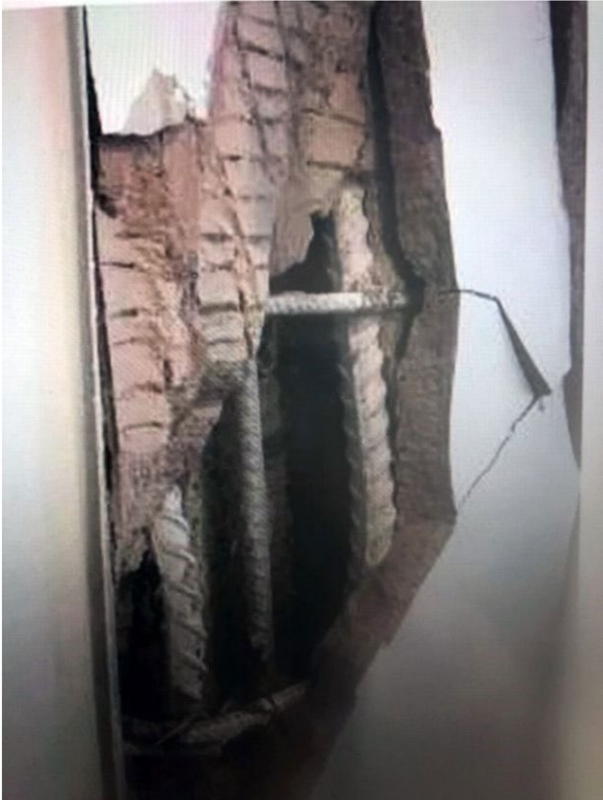
An image purporting to show steel rods within the fabric of the Victoria Square apartment block
