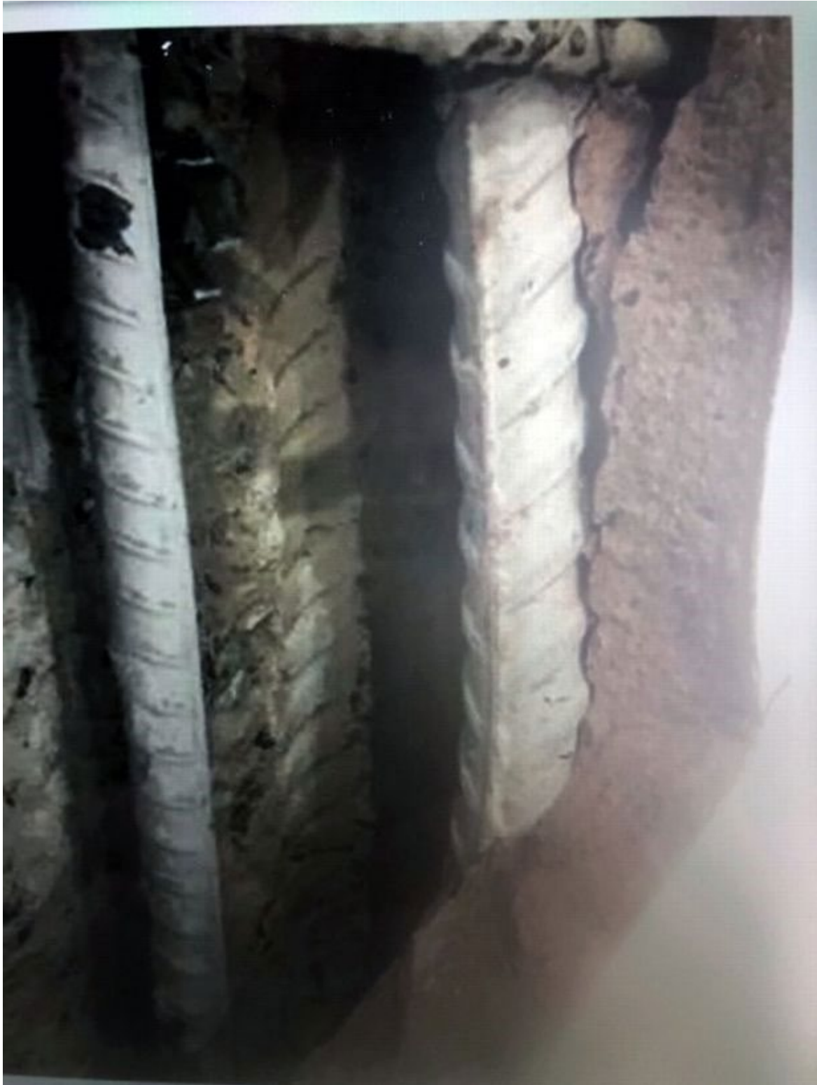
Another image of steelwork within the Victoria Square apartment block According to the source the cost-sharing proposal was turned down on that basis.
