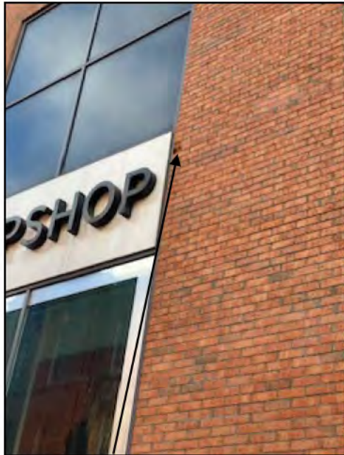
Reports of spalling brickwork
