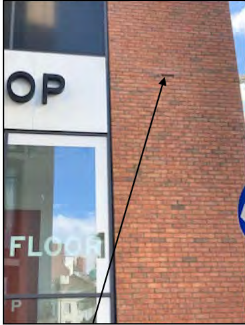
Reported spalling of brickwork
